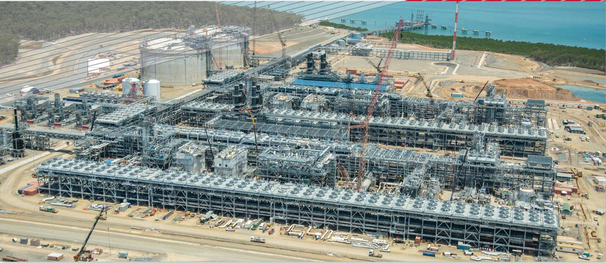
QCLNG Plant, Curtis Island, Queensland
