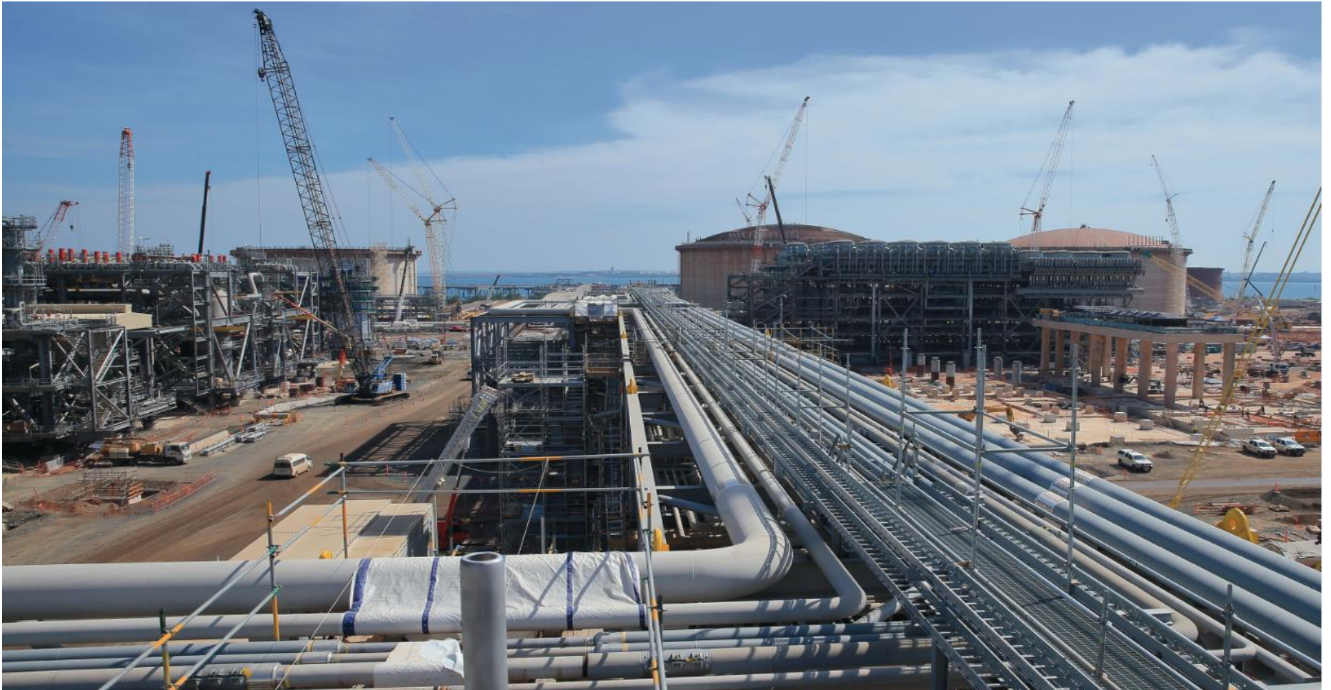
Ichthys Onshore LNG Facility, Darwin, Northern Territory
