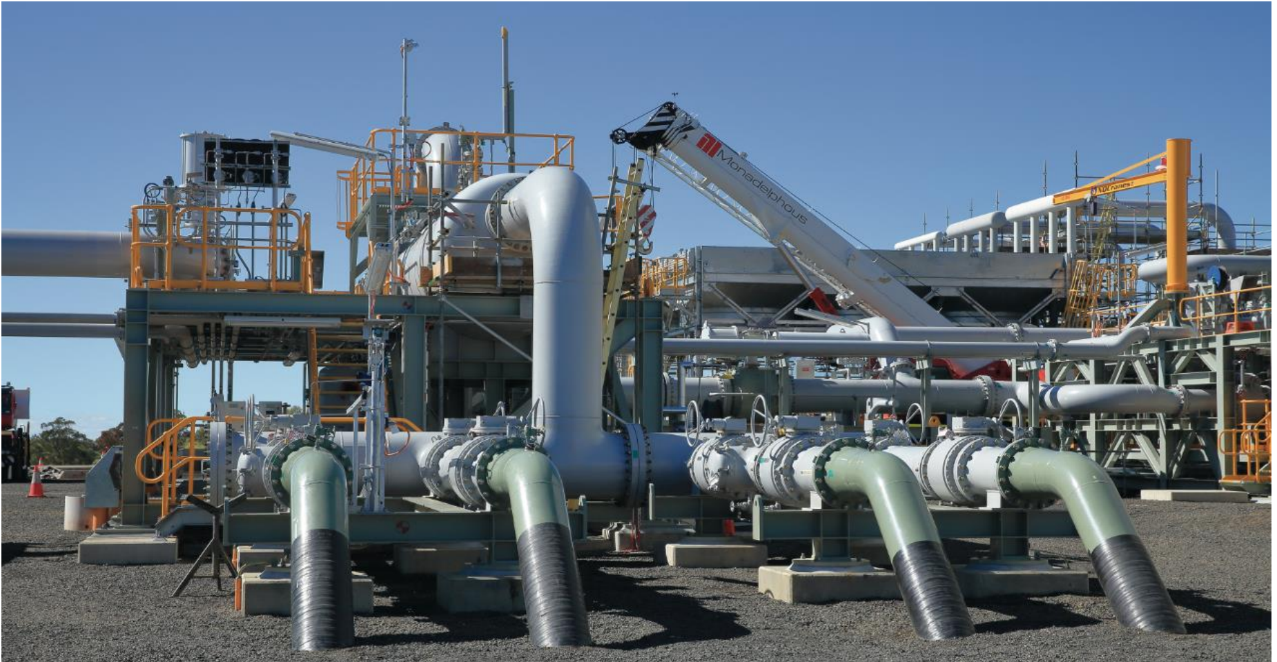
Eurombah Creek Gas Processing Facility, Queensland
