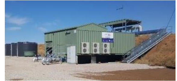
Pump station operational
