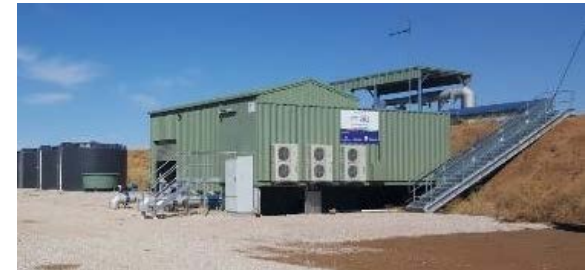
Pump station operational
