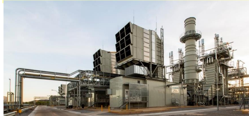
Diamantina Power Station – Power Block 1 (of 2)
