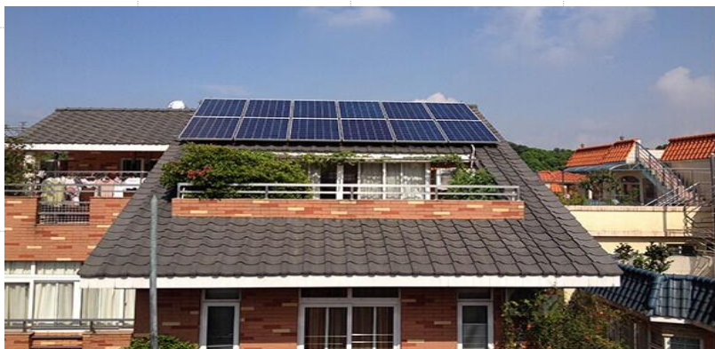
Rooftop solar power now commonplace, especially in rural areas
