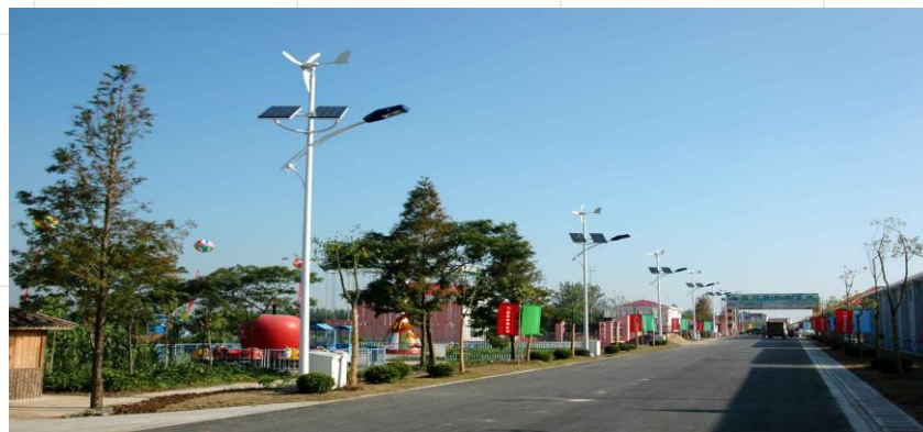
Standalone LED street lighting, powered by renewable energy
