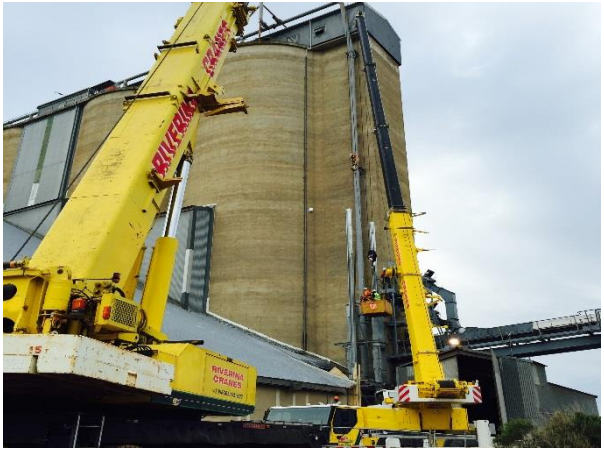
New bespoke elevator Junee Sub, SNSW
