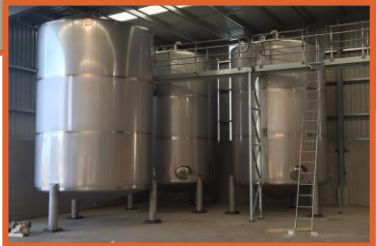
Tallow storage tanks
