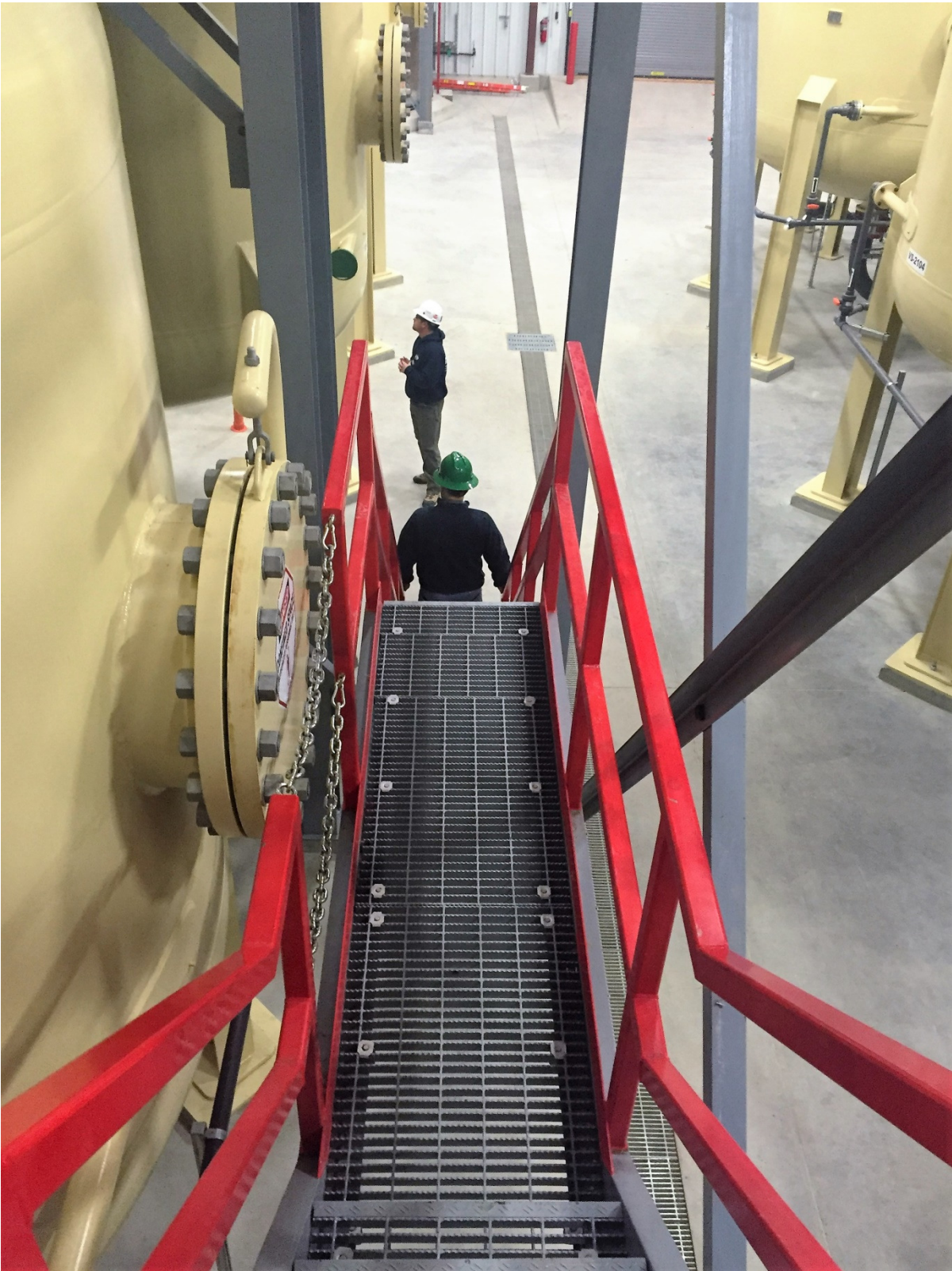
Figure 4: Ion Exchange Columns inside CPP, Lance Projects – April 2016
