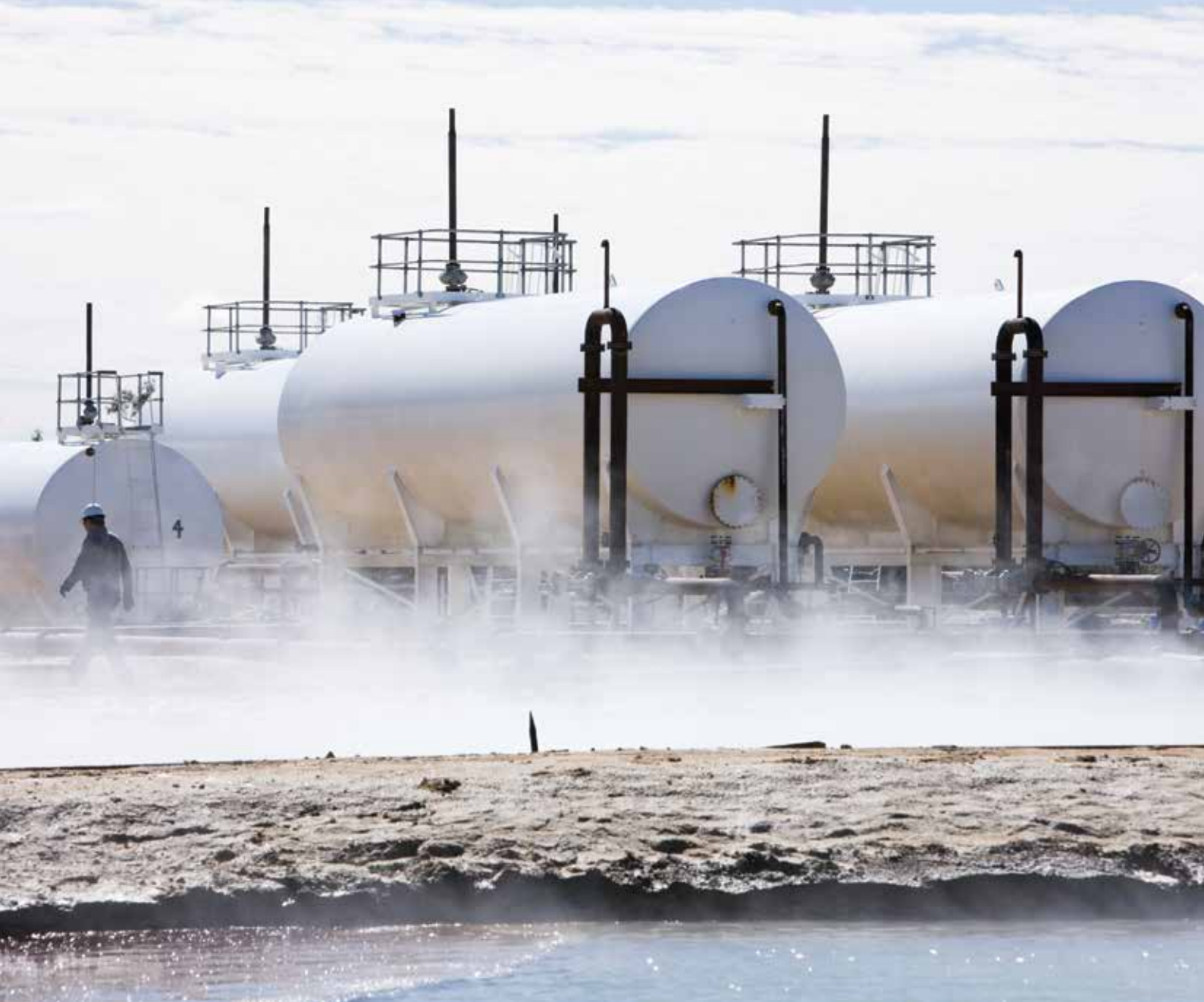
Oil tanks, Callawonga, Cooper Basin
