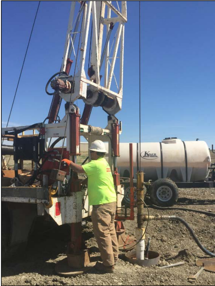
Figure 4-25: Swabbing of injection wells involves water blasting under pressure of screen to remove mineral precipitates
