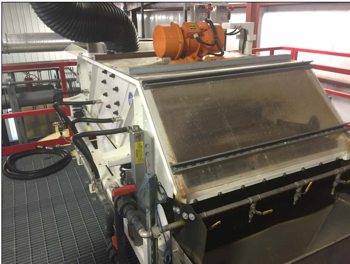
Figure 4-34: Screens installed to clean up PLS prior to ion exchange removal of uranium
