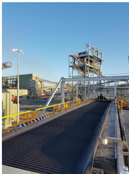
Filter Belt Commissioning
