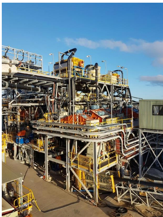
DMS Plant Reaches Mechanical Completion
