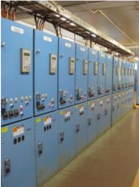
Power Room Isolate Electrical Power
