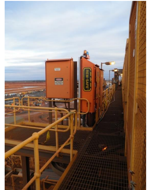
REMSAFE Field Isolation Station
