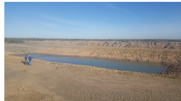
Mutton Hole cattle station, Gulf of Carpentaria (November 2016) New dam excavation. The development of additional watering points can provide access to previously unused grazing land
