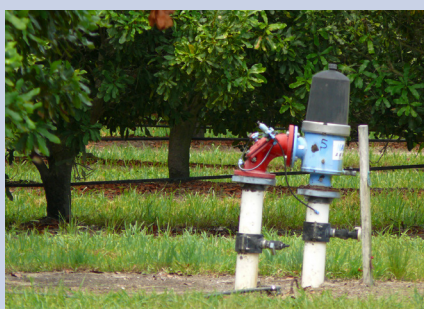
Automated irrigation infrastructure delivers water to macadamia orchards
