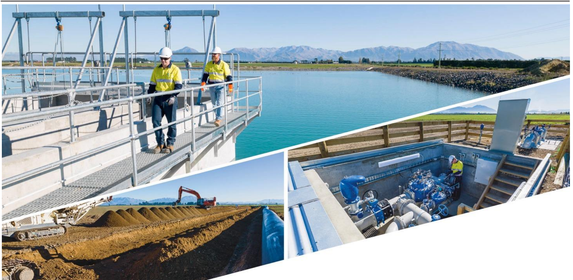
Ashburton Lyndhurst Irrigation Scheme (ALIS), South Island, New Zealand
