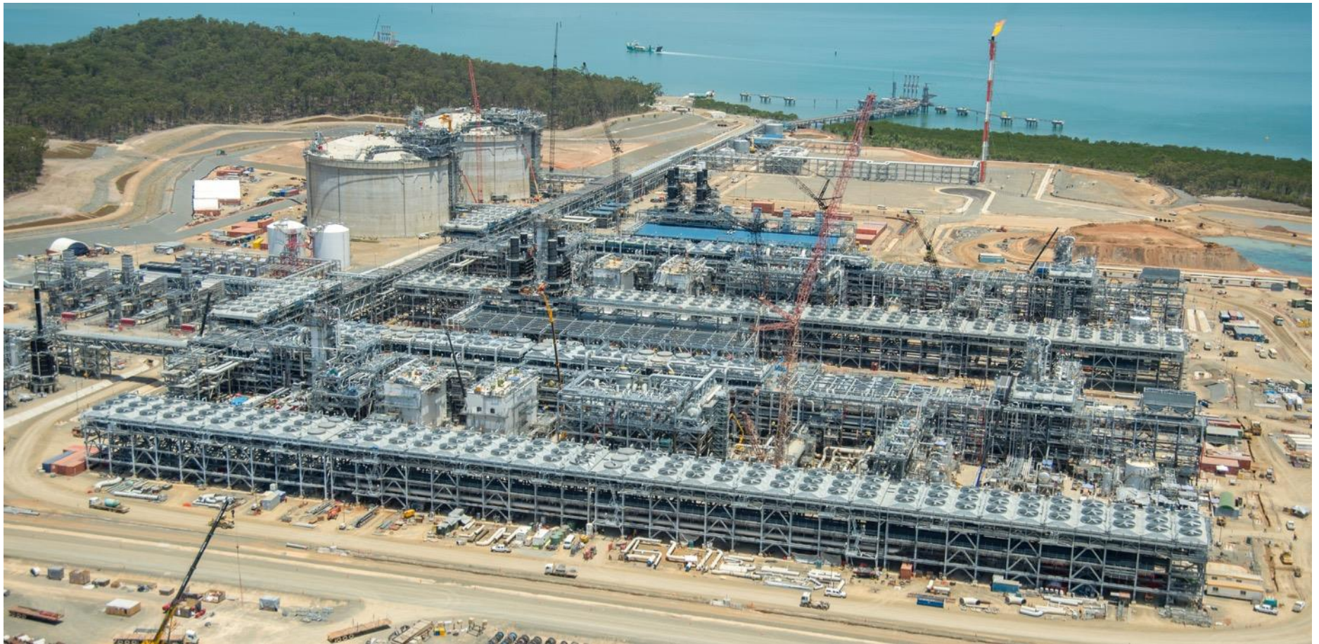
QGC plant, Curtis Island, Queensland
