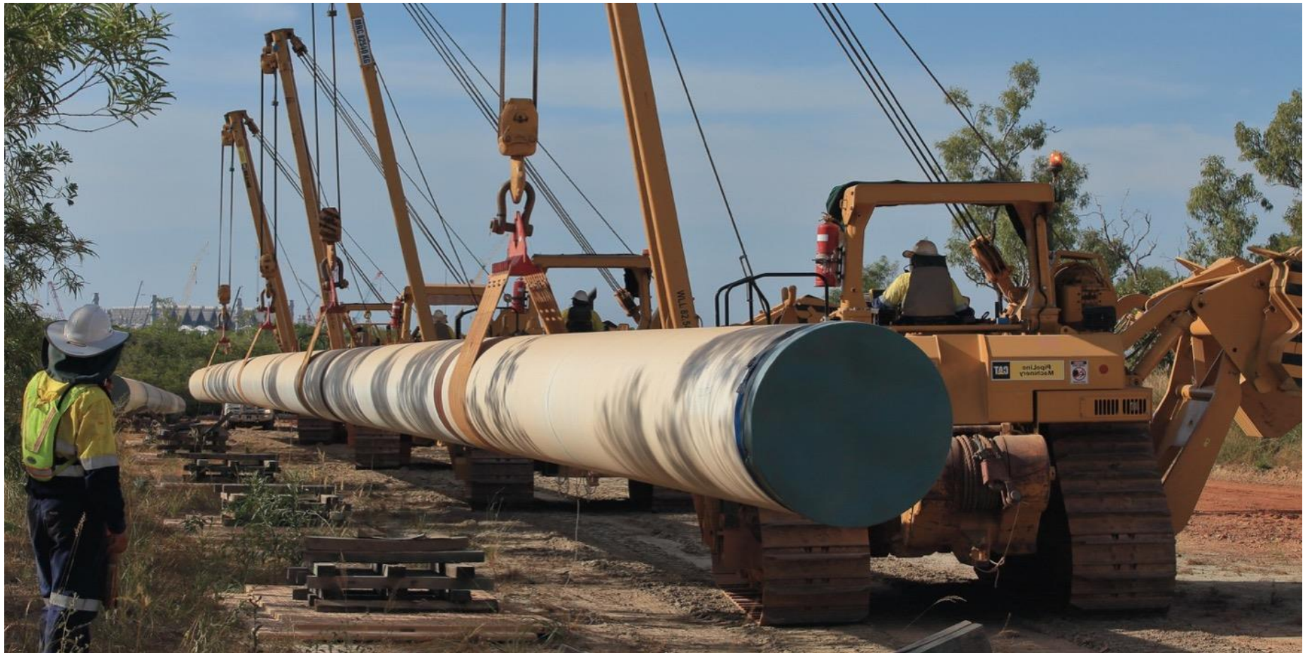
Relocating gas export pipeline 'string' at the Inpex-led Ichthys Project Onshore LNG Facilities, Darwin, Northern Territory
