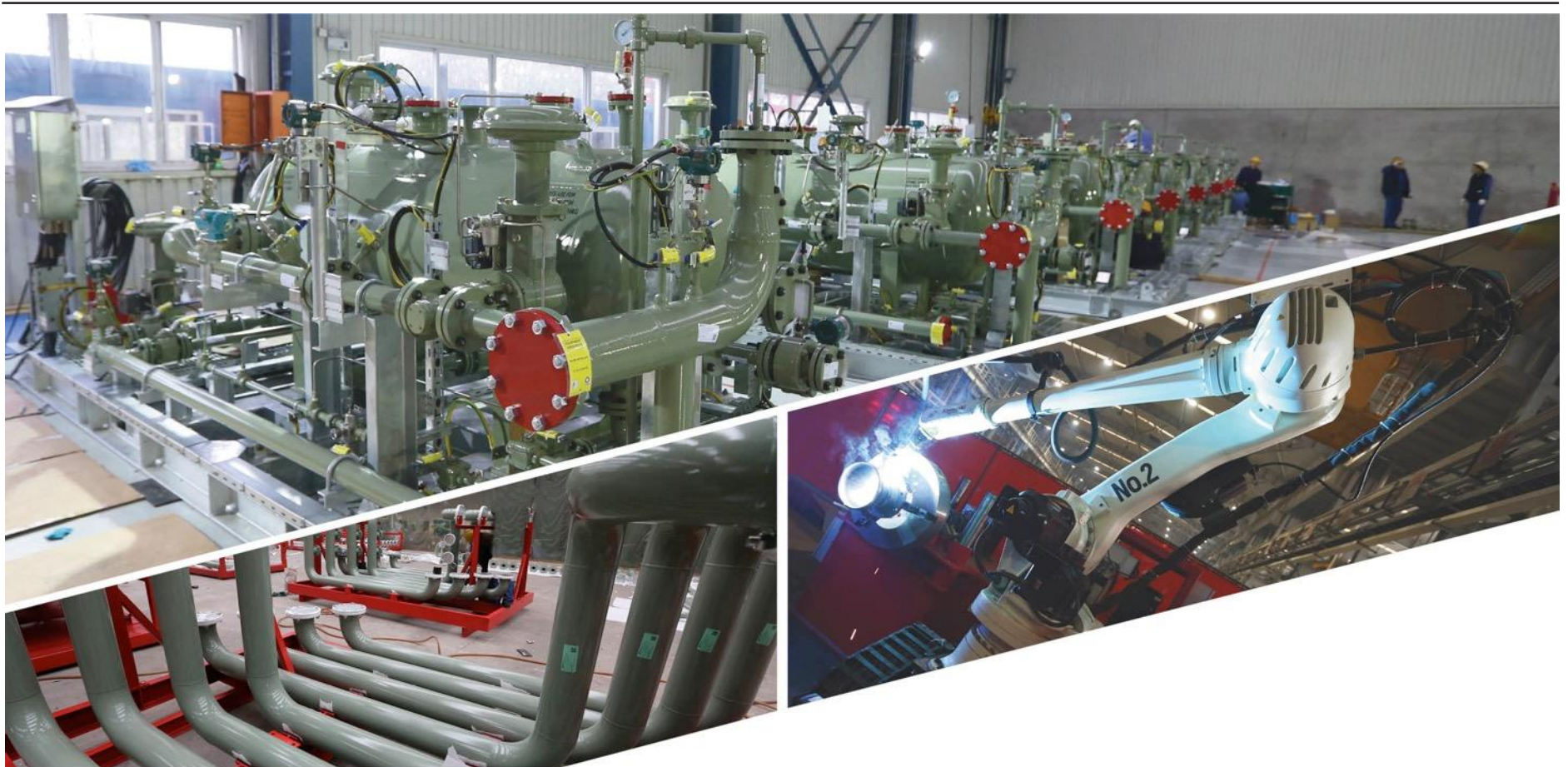
Well head separator skids, pipework and one of five welding cells commissioned at SinoStruct in China
