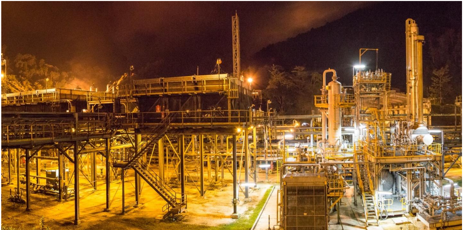
Oil Search Limited's Central Production Facility, Southern Highlands Province, Papua New Guinea
