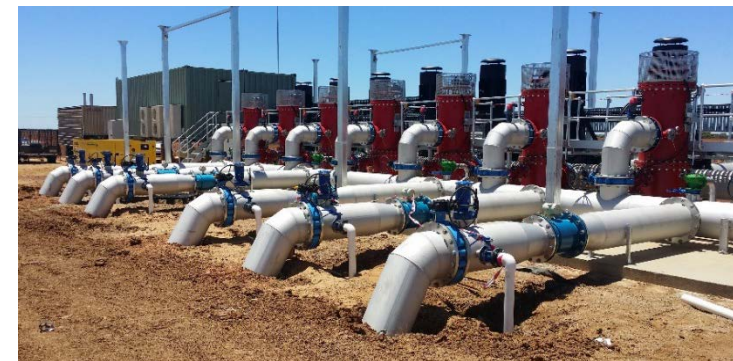
First pumping station for Kerarbury. Pumps can deliver 2,400 litres per second to the orchard. Image taken Dec 2016
