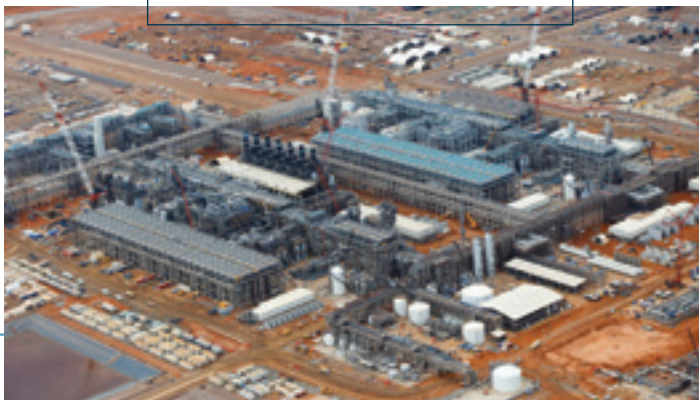
All Wheatstone Project Train 1 and Train 2 modules are set on their foundations.
