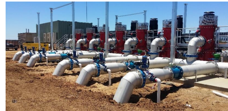
First pumping station for Kerarbury. Pumps can deliver 2,400 litres per second to the orchard. Image taken Dec 2016
