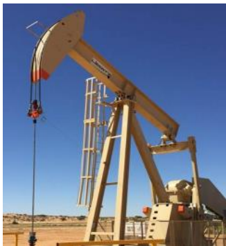
Variable speed beam pump installation in ex PEL 91
