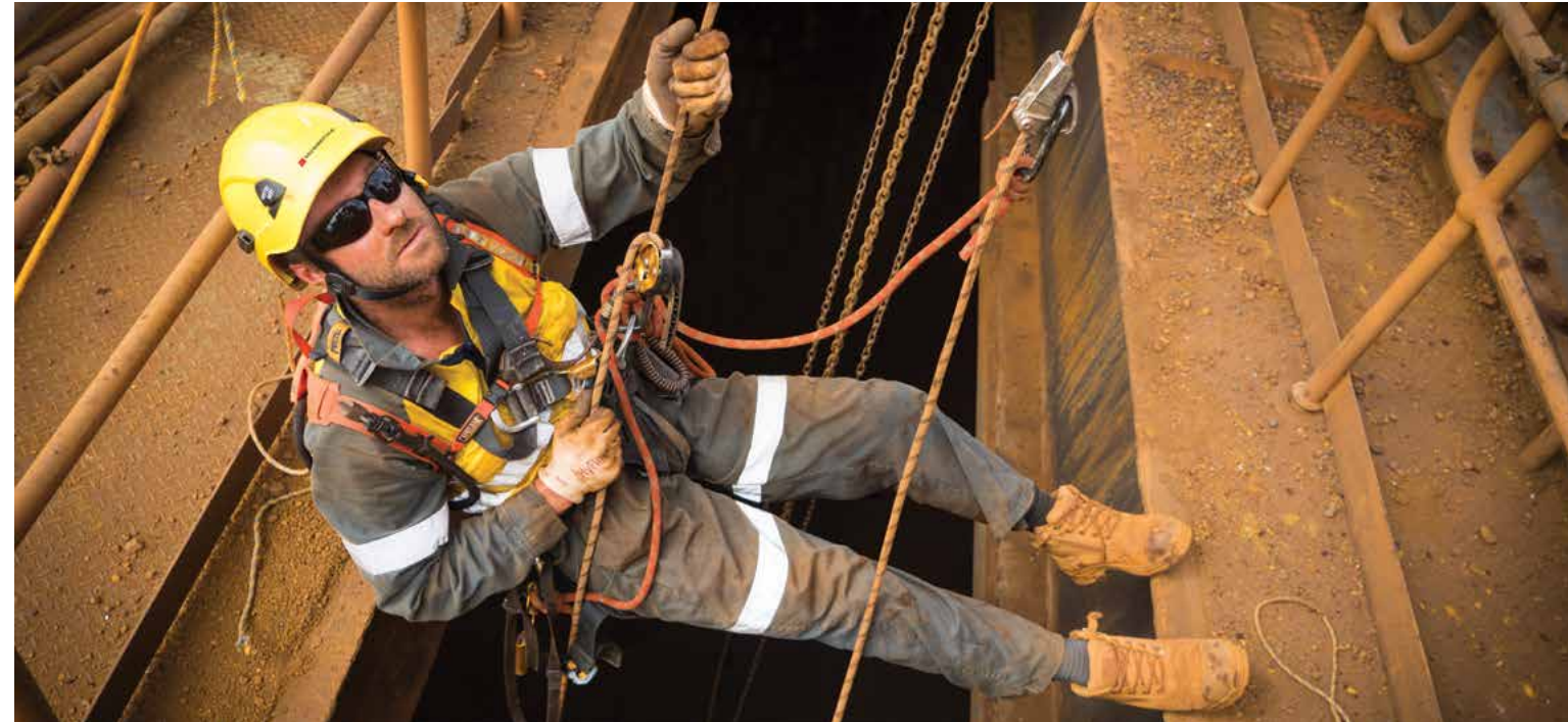
IMAGE A member of the Monadelphous rope access team entering a train loadout bin for inspection at BHP's Mining Area C, Newman, Western Australia.
