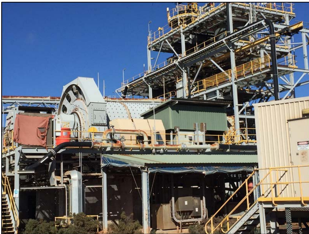
Figure 1: Black Swan Grinding Circuit (10MW of installed power)
