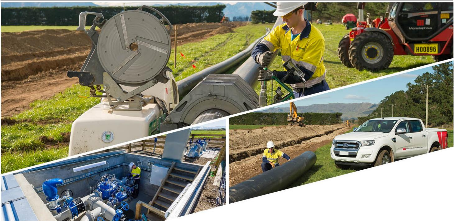
Amuri Irrigation Scheme and Ashburton Lyndhurst Irrigation Scheme, New Zealand
