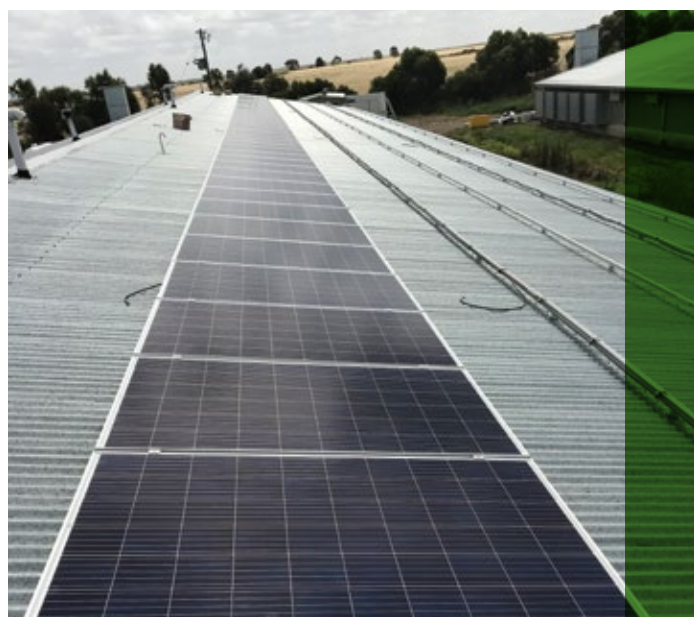
Recently installed solar panels on the roof of poultry sheds, Lethbridge, Victoria, December 2017
