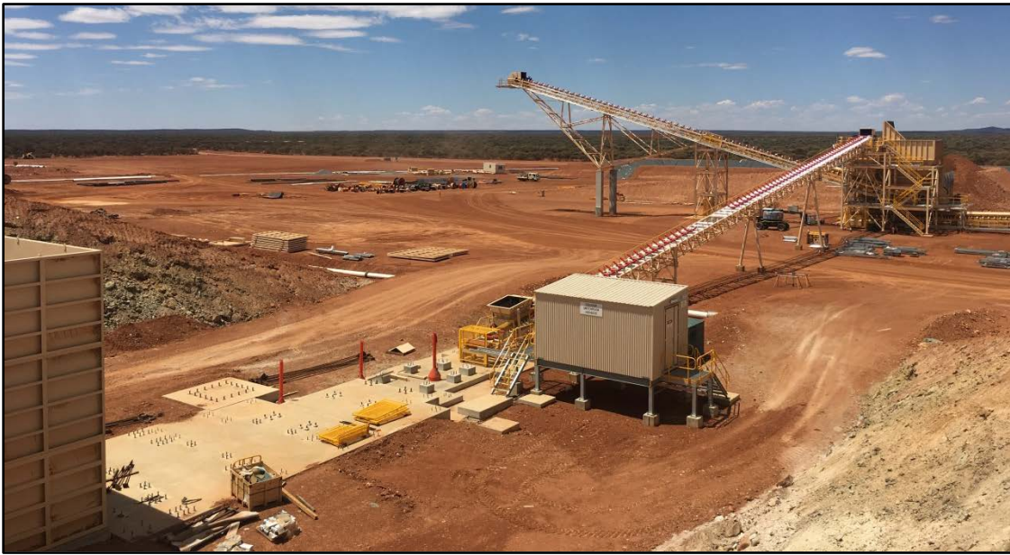
Photo 2: Crusher Foundations and MCC, along with Main Feed Conveyors and Ore Transfer Bin
