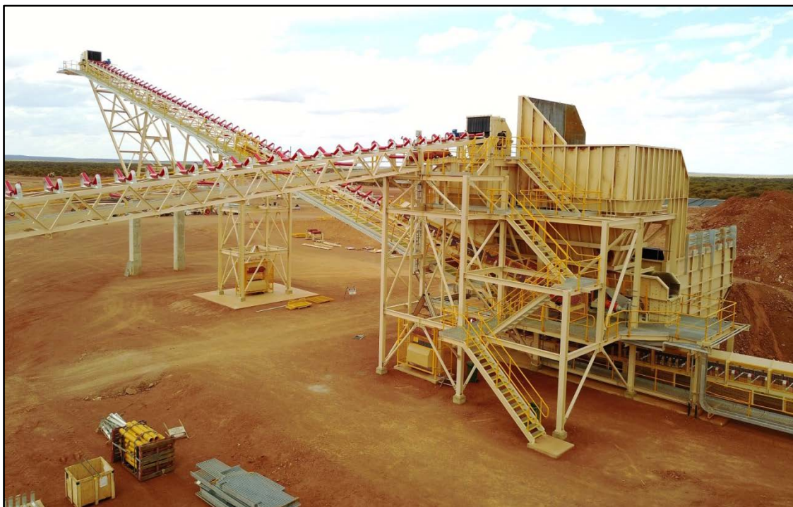
Photo 3: Ore Transfer Bin, including Feed and Stockpile Conveyors
