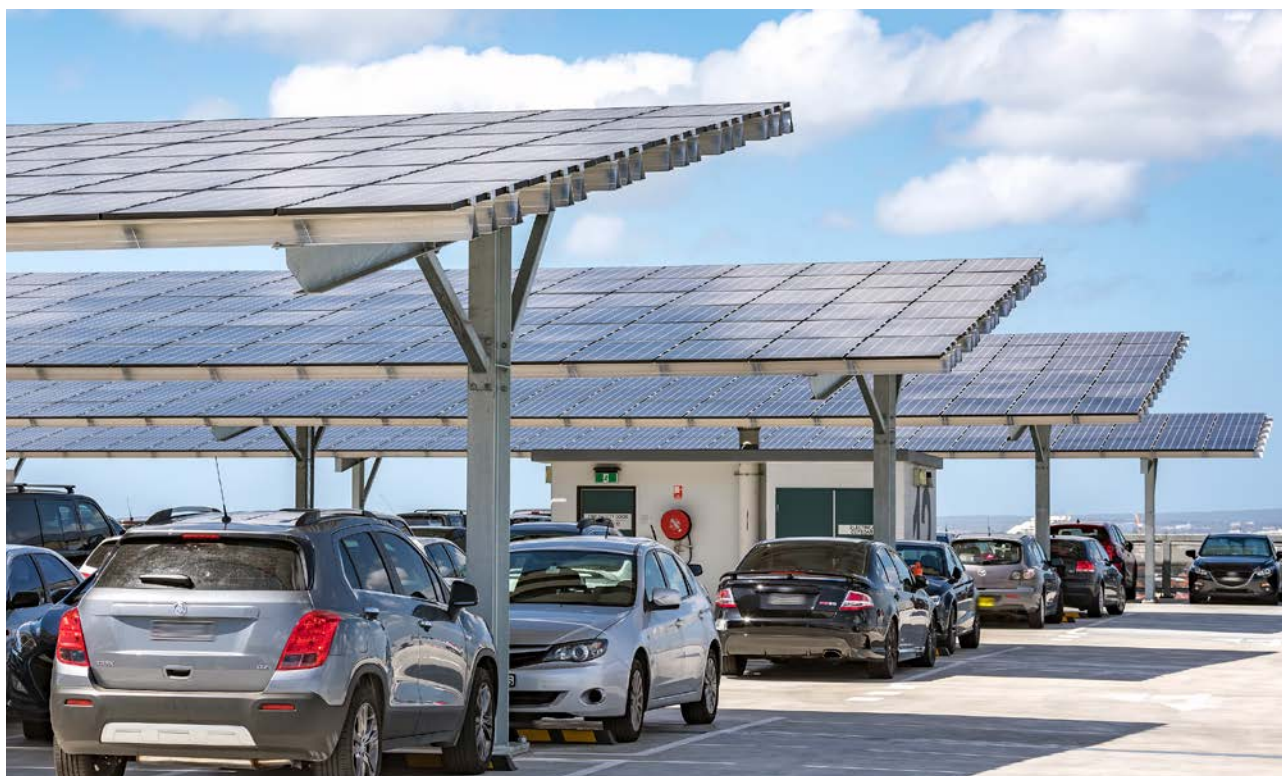
The solar panel installation at Sydney Airport's T1 International terminal car park.
