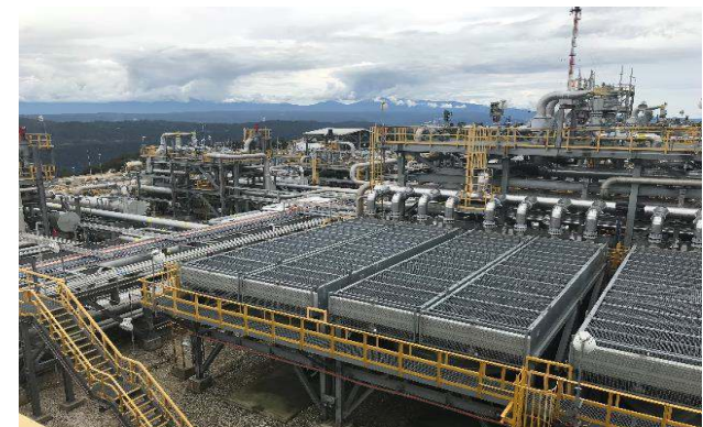
Hides Gas Conditioning Plant process area, 1 March 2018
