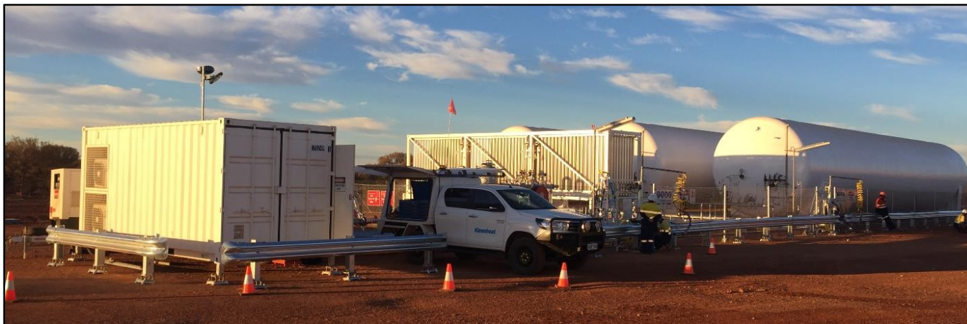
Photo 11: Commissioning underway of the LNG Storage and Vaporisation Facility
