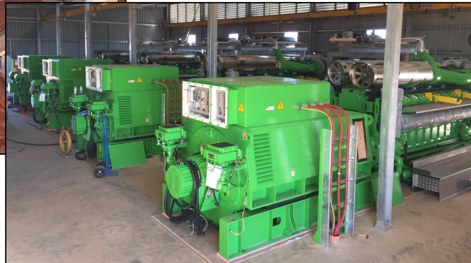
Gas Generators – Installation Well Advanced
