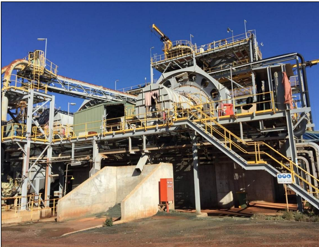
Figure 3: Black Swan Process Plant
