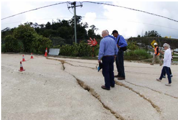
Damage at the entrance to Ridge Camp
