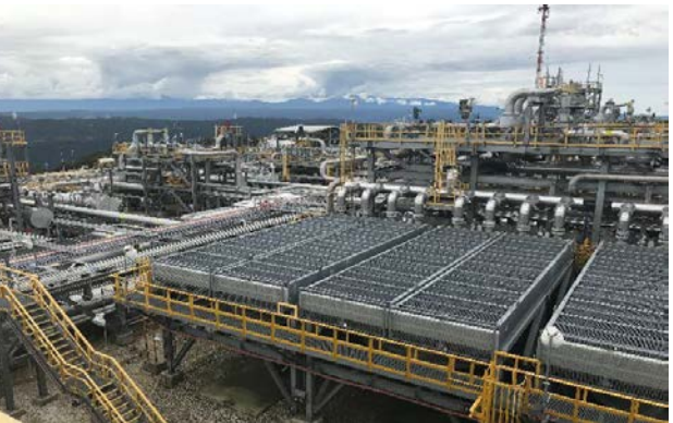
Hides Gas Conditioning Plant process area, 1 March 2018
