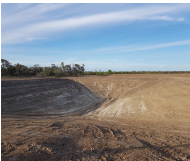
New water storage on Natal, northern Queensland, January 2018.
