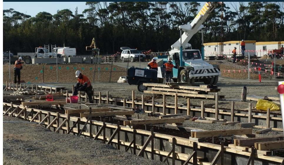
APA Group: plant upgrade
