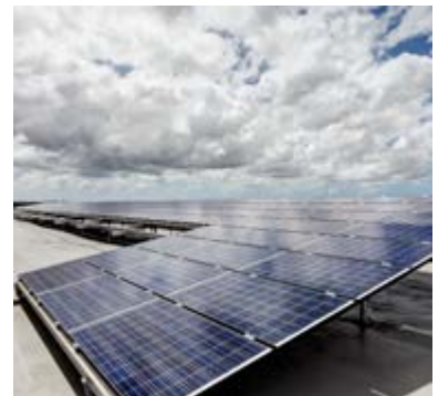
A total of 175MWh of solar energy was generated during CY17 from 5 Murray Rose Avenue, Sydney Olympic Park, NSW
