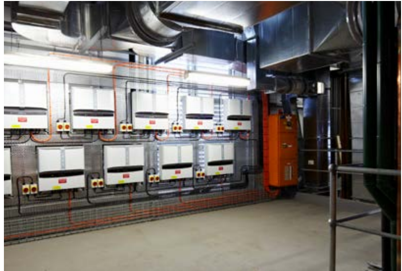
Solar inverters at 5 Murray Rose Avenue, Sydney Olympic Park, NSW
