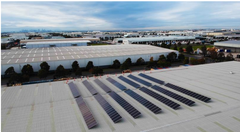
34 West Park Drive, Derrimut – 100kW solar installation
