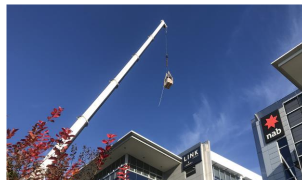
Solar installation (Building A, Rhodes)
