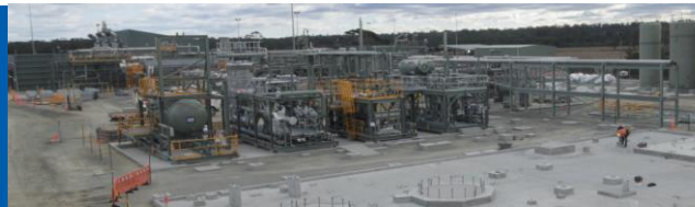
Orbost Gas Plant: Inlet gas area
