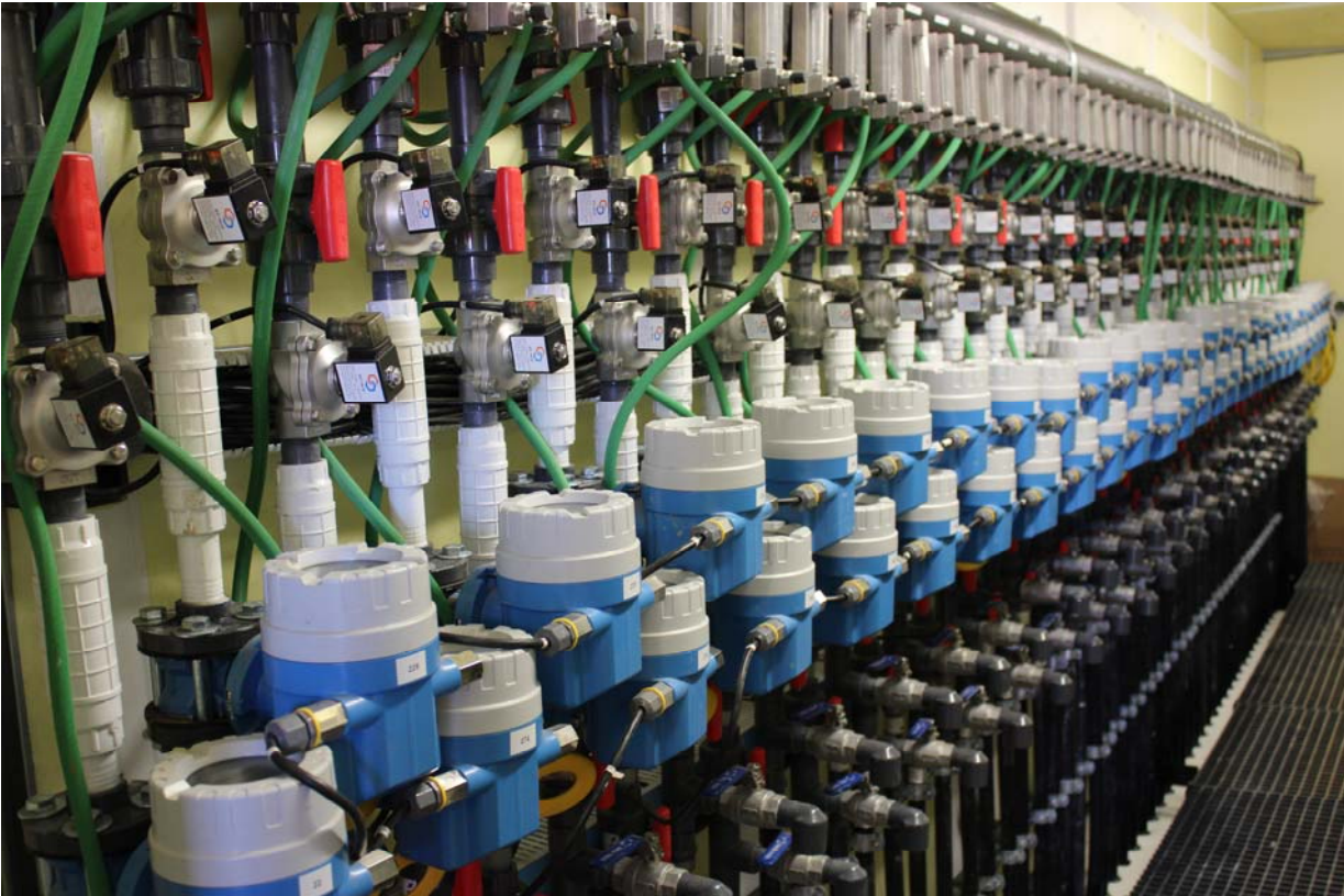
Figure 4: Header House Interior, Lance Projects, Wyoming USA
