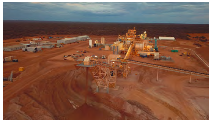
Photograph 2: Process plant commissioning May 2018
