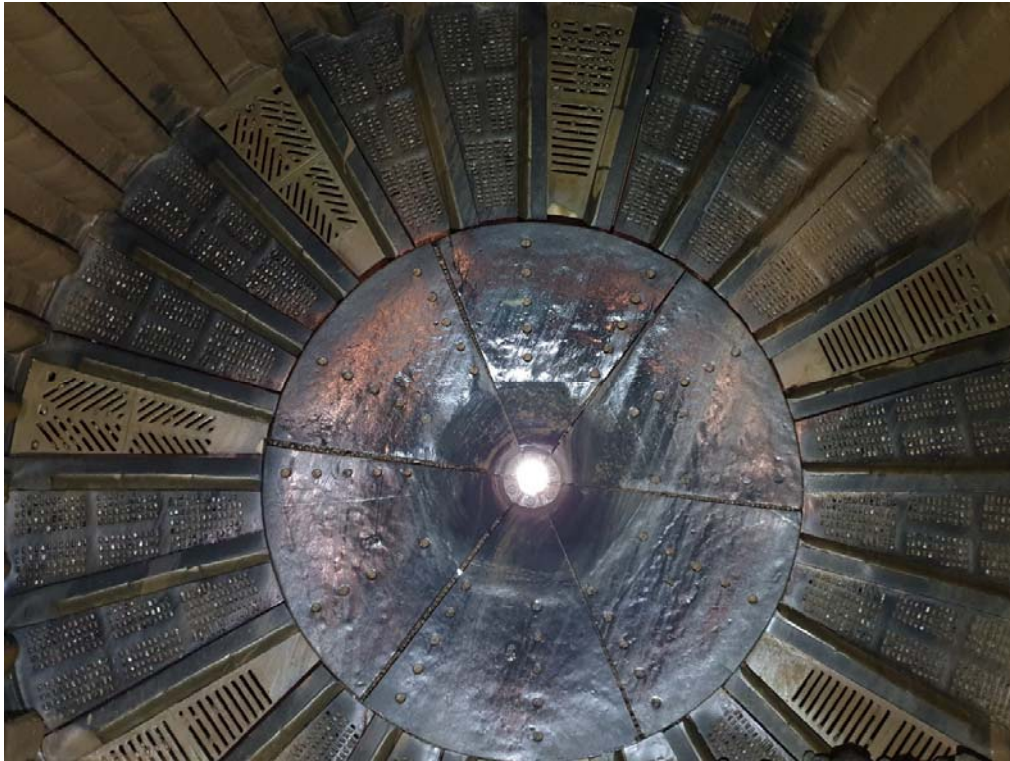
Figure 2; Photograph taken 2 weeks after hardox grate installation, with hardox grates essentially clear and the rubber grates almost completely pegged.
