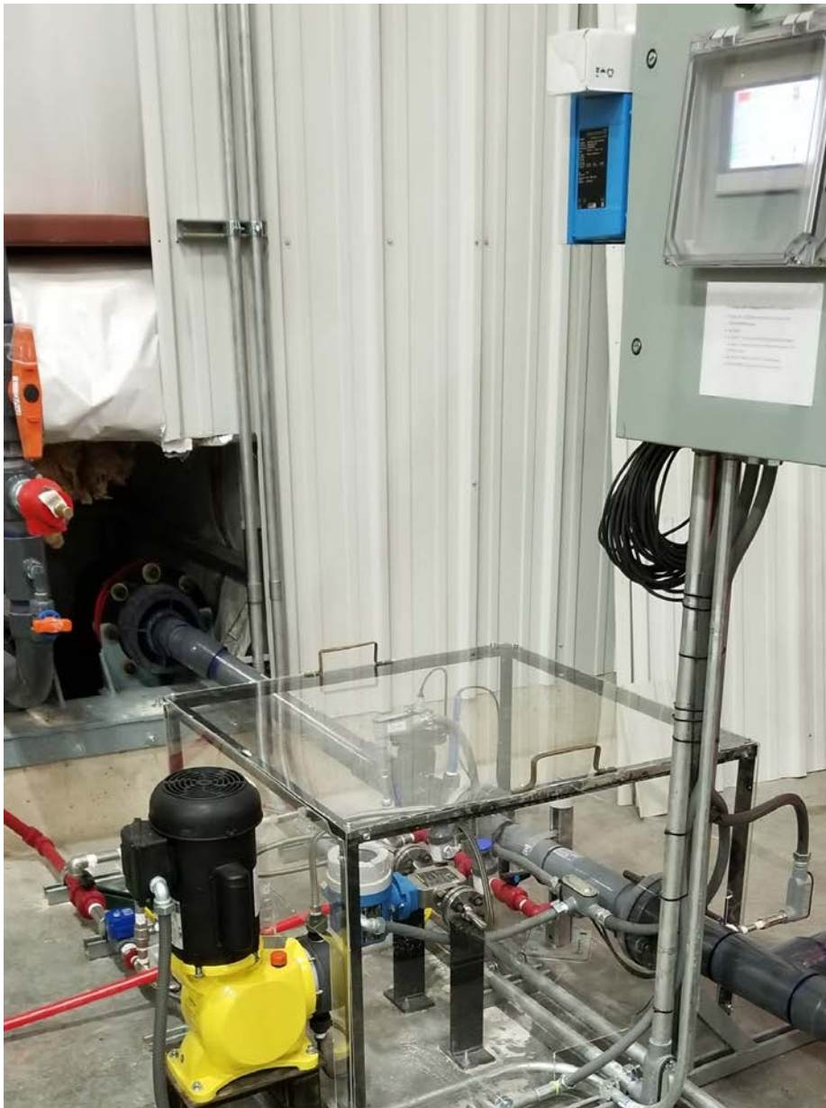
Figure 2: Low pH Field Demonstration - acid dosing pump, Lance Projects, Wyoming USA
