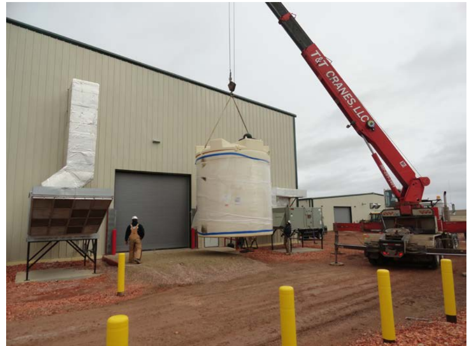
Tank for low pH field demonstration
