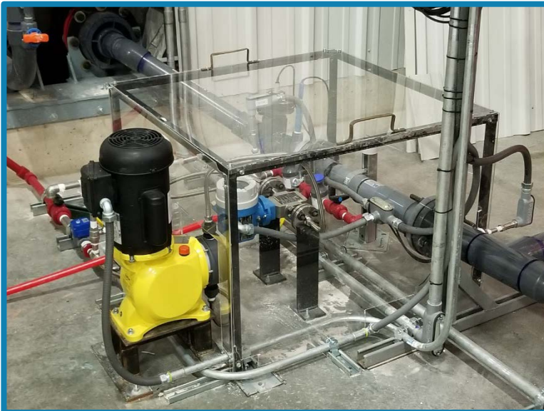
Sulfuric Acid Addition Pump
