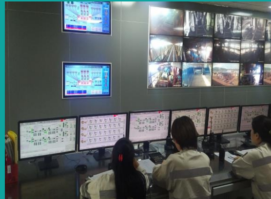
RKEF Control Room
