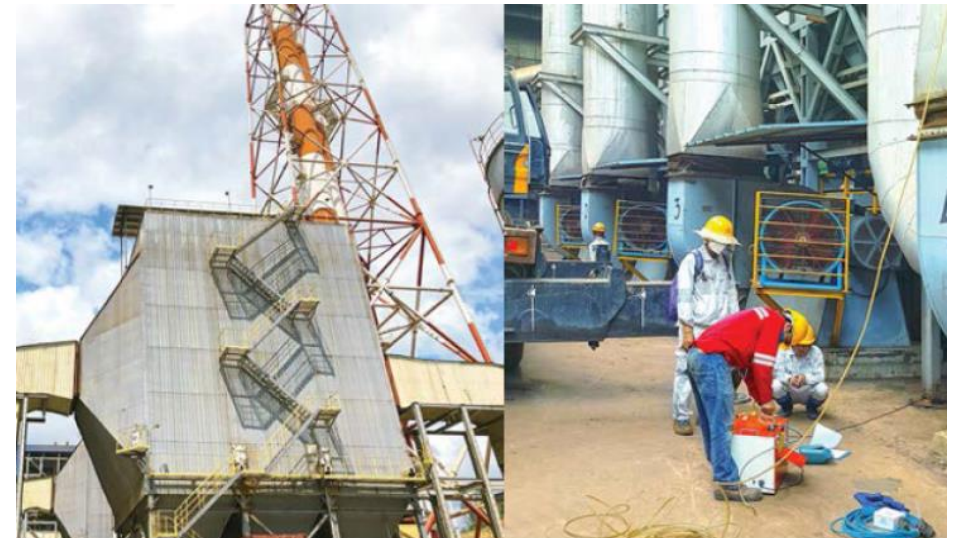
ESP Dust Collector (left) and official emission testing of dust collector at an RKEF smelter(right)
