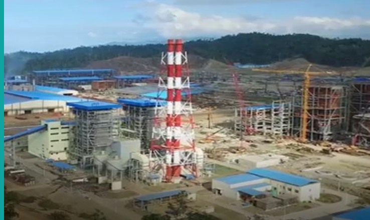
2GW Coal Fired Power Station
