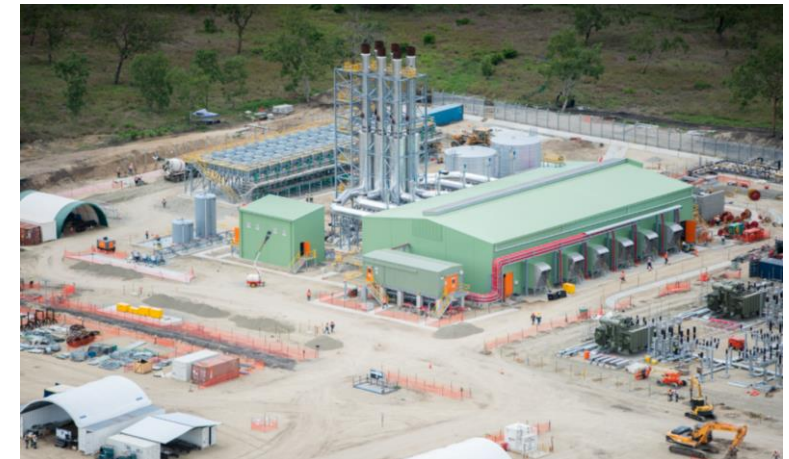
58MW gas fired power station, located adjacent to PNG LNG plant site.
