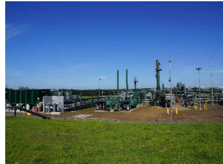
Minerva Gas Plant Currently owned by Minerva Joint Venture. To be acquired by Cooper Energy/Mitsui Joint Venture for processing Otway gas
