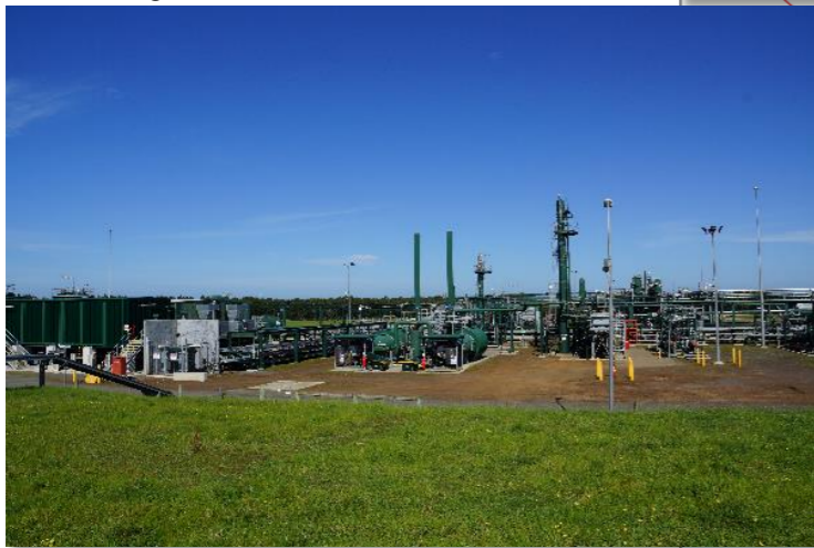
Minerva Gas Plant
