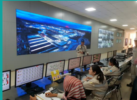
RKEF Control Room
