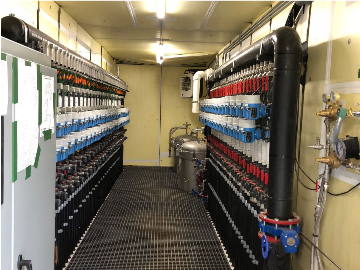
Figure 4: Header House Interior, Lance Projects, Wyoming, USA
