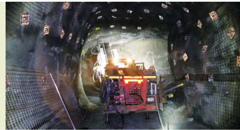
The first stage of the Silver Swan underground rehabilitation commenced on 25th February 2019 and ran to mid May 2019. The jumbo is pictured installing and replacing mesh in key areas of the mine.
