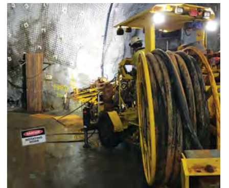
A total of 3,662 metres of diamond drilling was performed at the bottom of the Silver Swan decline between March and June this year.
