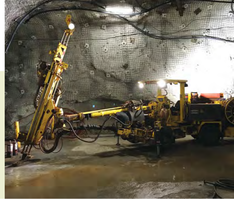
Jumbo mounted diamond drill rig which allows exceptional flexibility in an underground environment.
