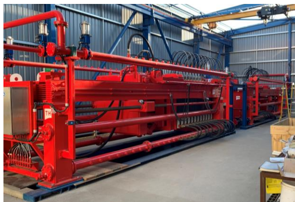
Lead/Zinc Filter Press in Filter Building
