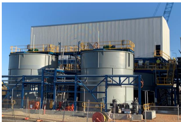
Dewatering & Filter Building
