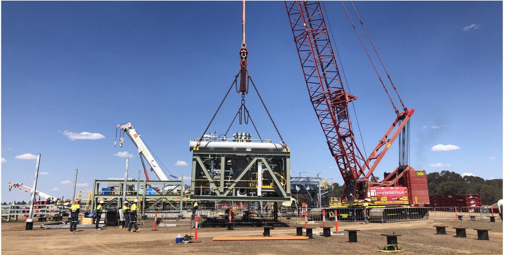
Talinga Orana Gas Gathering Station near Chinchilla in Queensland.
