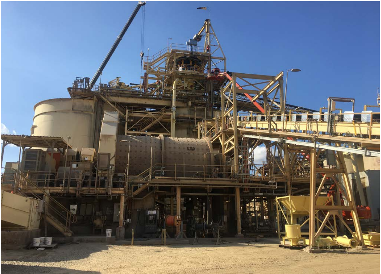
Figure 1: Nolans Processing Plant with third grinding mill (Mill #3)
